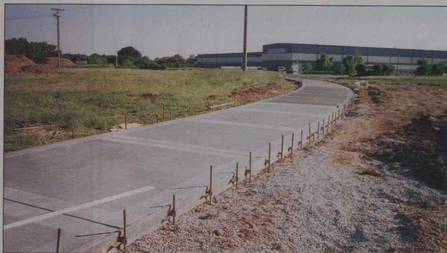
Poly Meta Forms are still in place on this sidewalk pour. Note their clean and simple construction and the lack of backfill or bracing.
